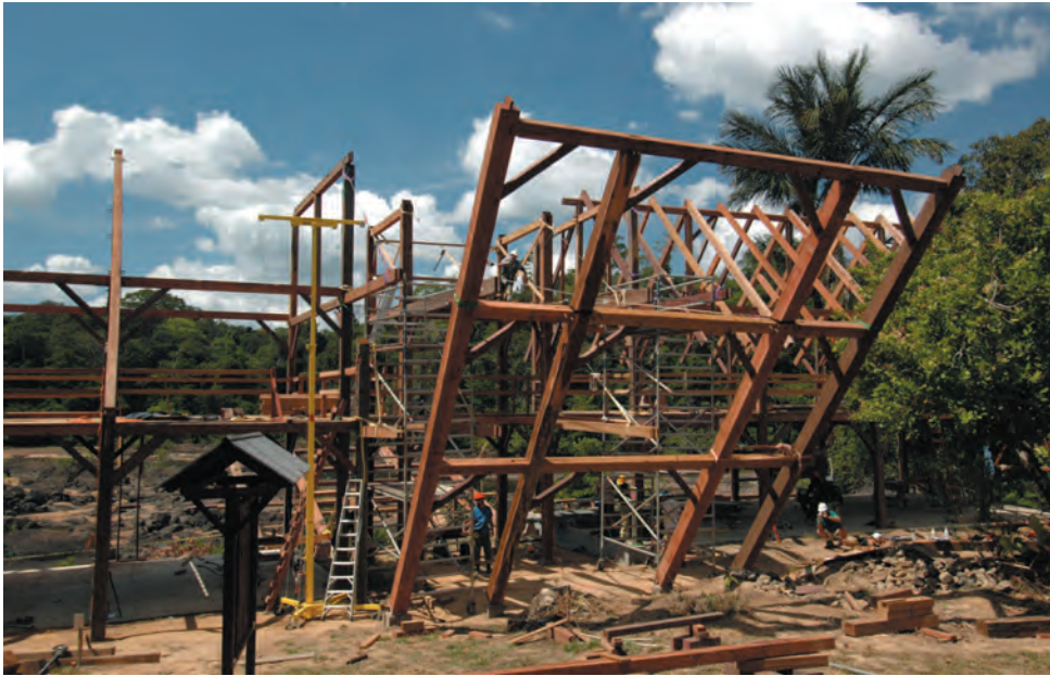
Fig. 6. Mid-raising, a 12,800-lb. frame for the central section is pulled into place.
