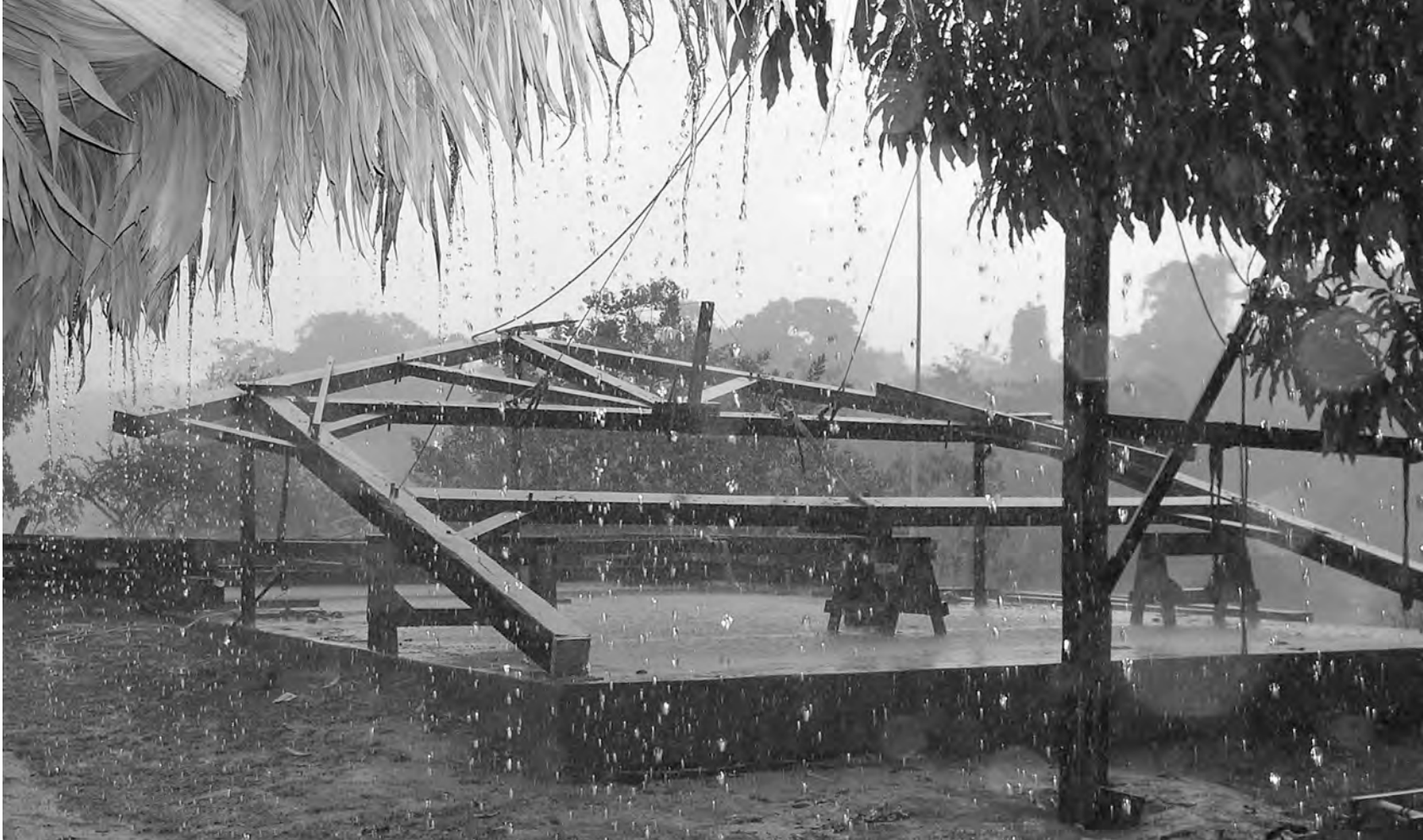
Fig. 5. Assembled end-bent readied for raising via winches pulling over unseen A-frame fulcrum. Note metal base for post foot.
